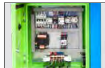
Control panel box.
